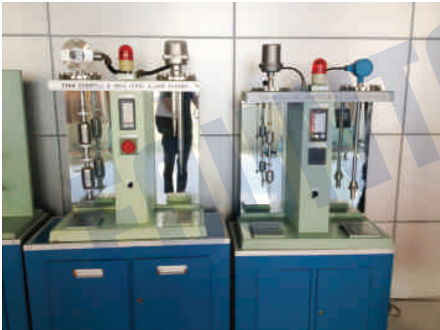
Tank Level Alarm System
