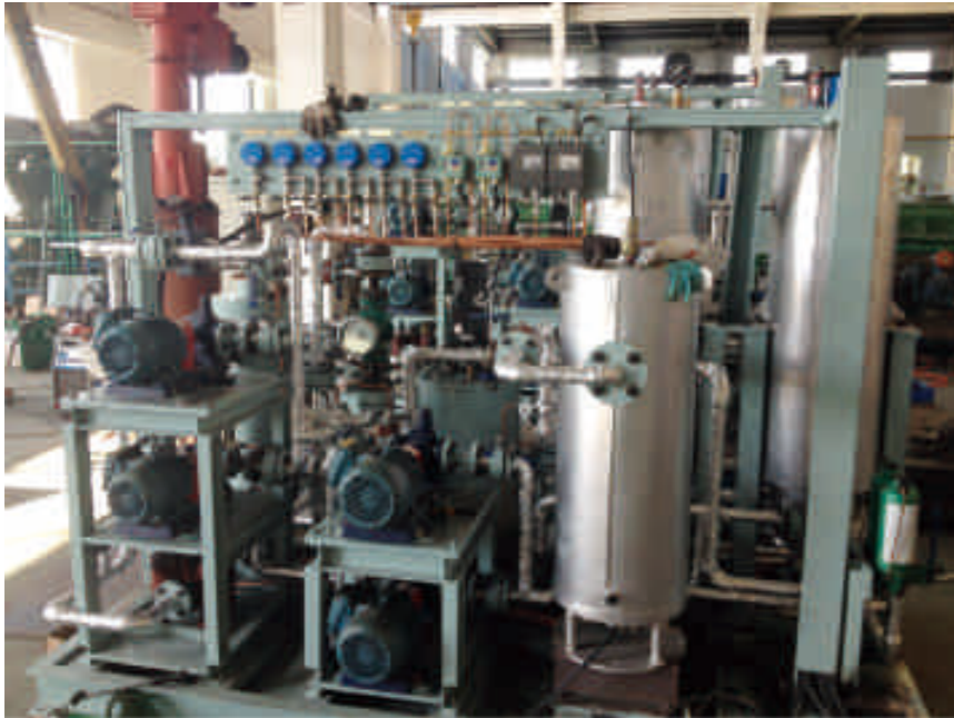
Fuel Oil Supply Unit
